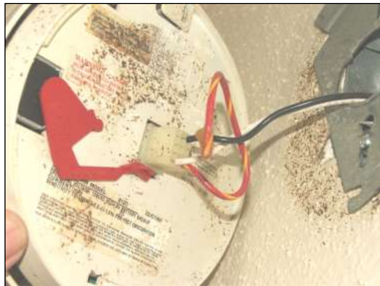
Cockroach infestation in a smoke detector
