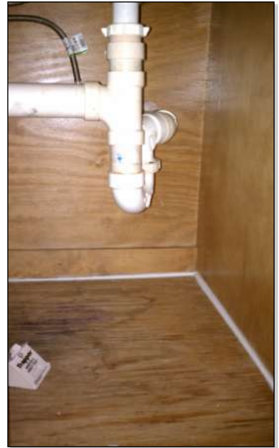
Monitor under a well-sealed sink
