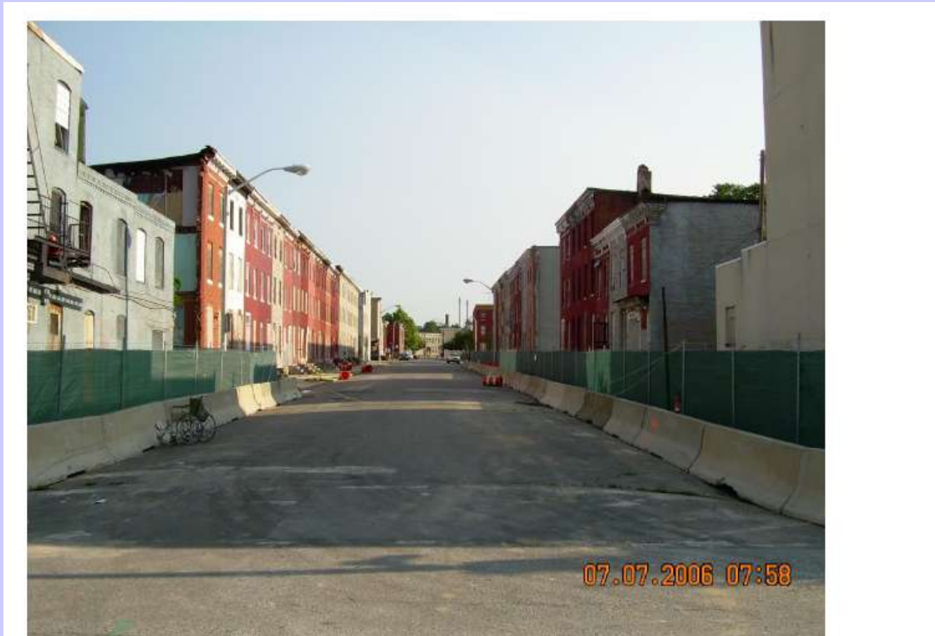
Photo 16: Image taken at the 1700 block of E. Eager Street and 1000 block of McDonough Street intersection. View from south to the north.
