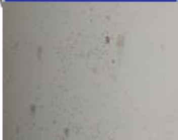
Water leaks creating mold hazards
