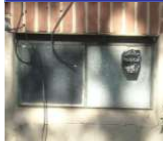
Deteriorated inefficient windows
