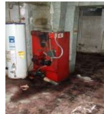
Broken hot water heater and furnace
