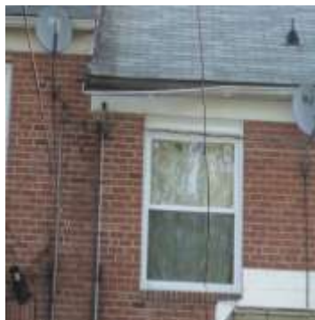
Defective gutters causing water leaks
